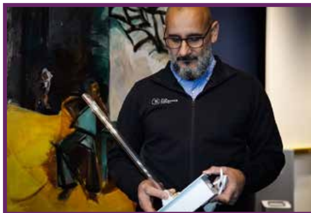
A Kool Concept Inc. Technician Installing their UVGi Air Purification System into the Central HVAC Units at The Exchange Hotel Downtown Sacramento.
